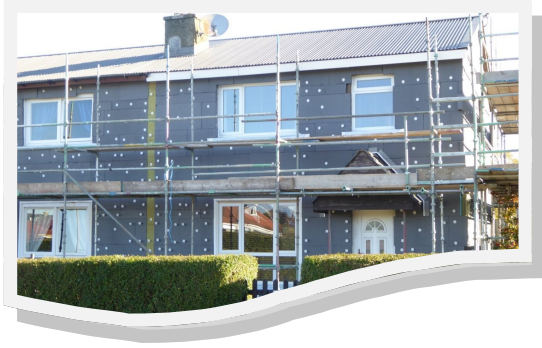
Fig 1 Insulation boards fixed to ground and upper floors of semi detached houses.
